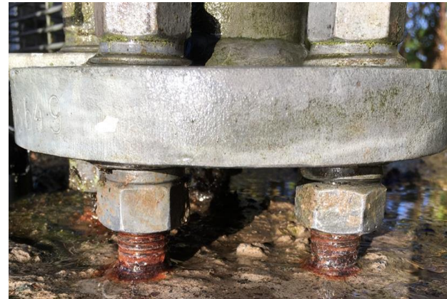
Corroded Hold Down Bolts.
