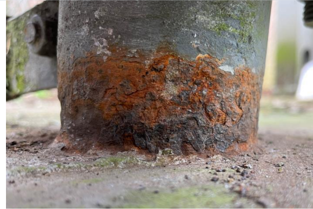
Corroded tubular legs (the internal space was also corroded).
