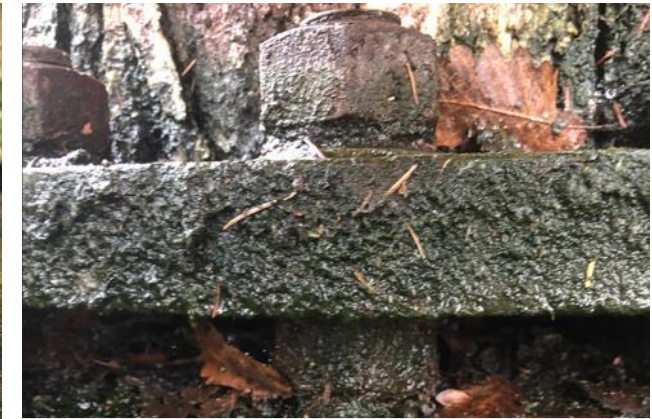
Build-up of Detritus with Corroded Nuts.
