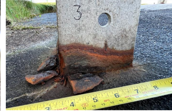
Corroded Angle Stubs.
